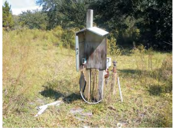
View of the an old power junction box
